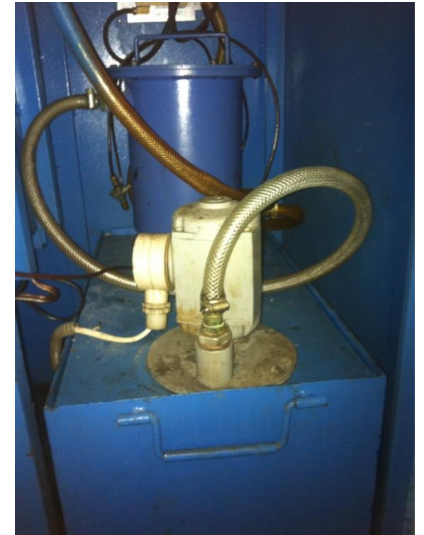
Lubrication Pump, Filter and Tank
